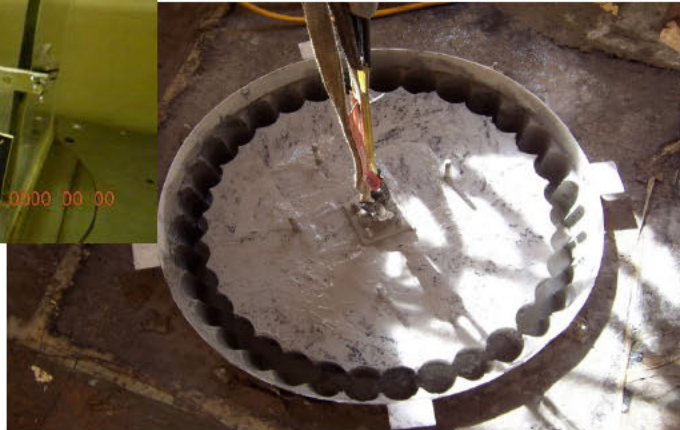
Three foot diameter access hole cut for insertion of Robot for H-Canyon Tunnel Inspection
